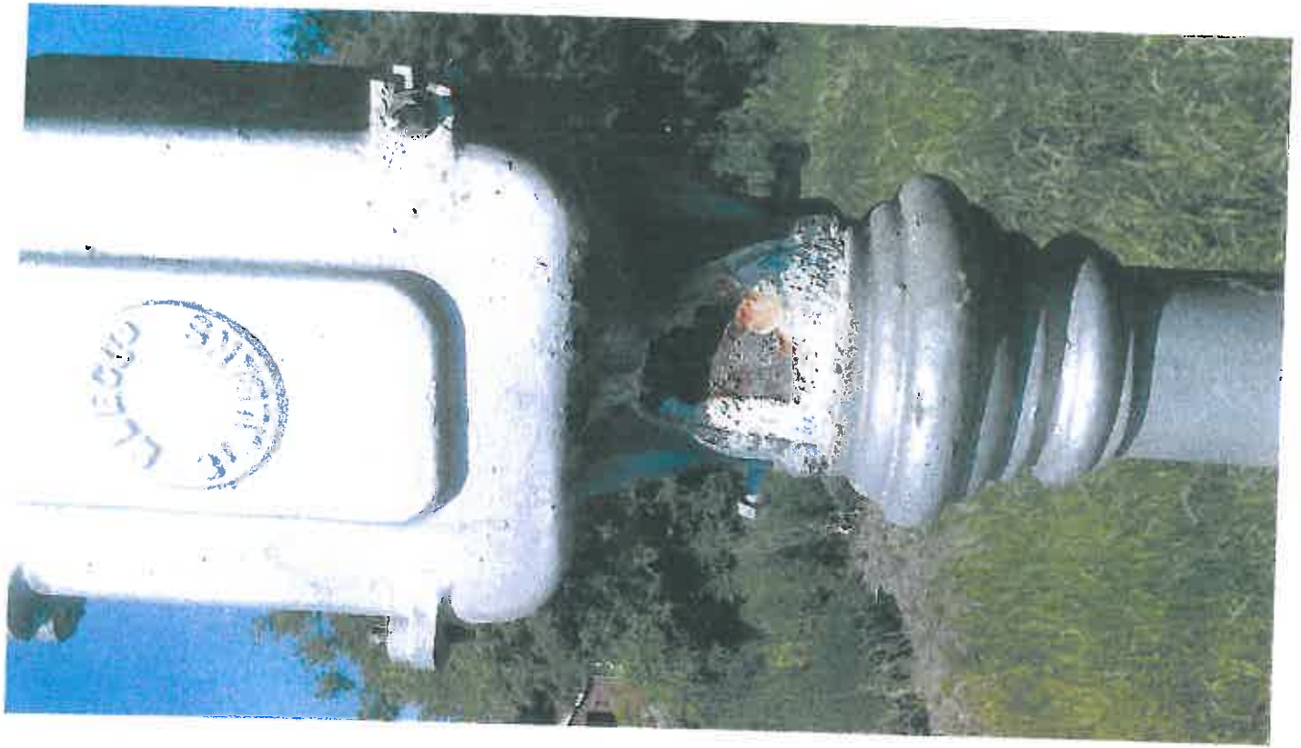
COLUMN ST, BROOK END BEESTON, TOP OF COLUMN SPIGOT CRACKED AND BADLY CORRODED.
